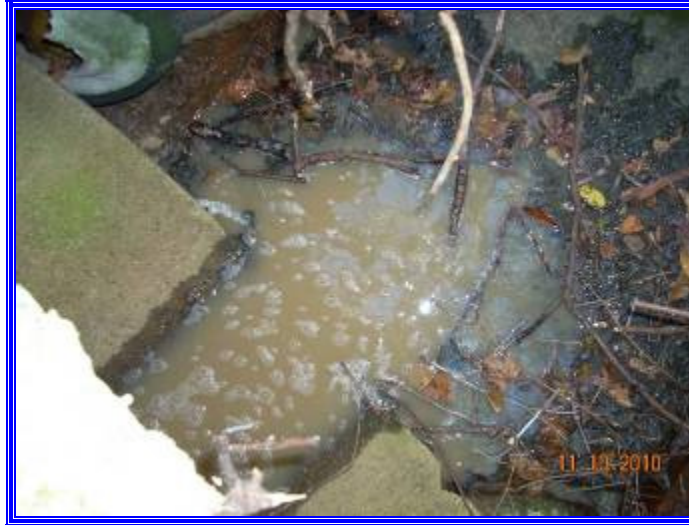
Figure 5.1: Sediment Discharge at Hendersonville Elementary.
