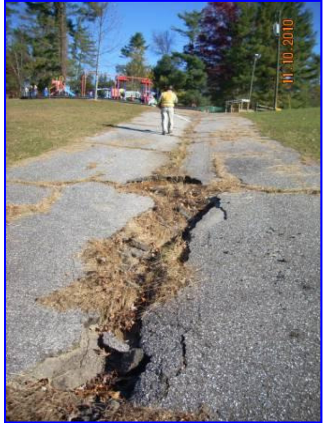
Figure 5.8: Asphalt Swale at Hendersonville Elementary.
