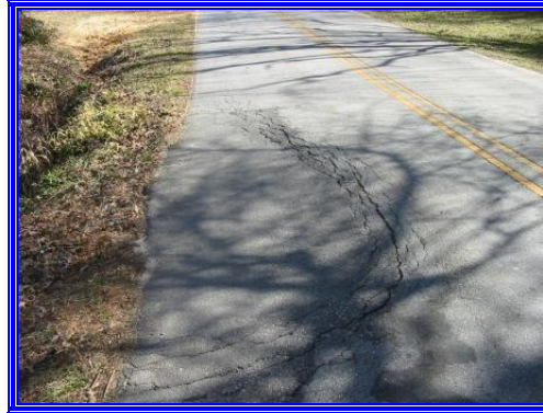
Figure 5.16: Sinking Asphalt on Long John Drive.
