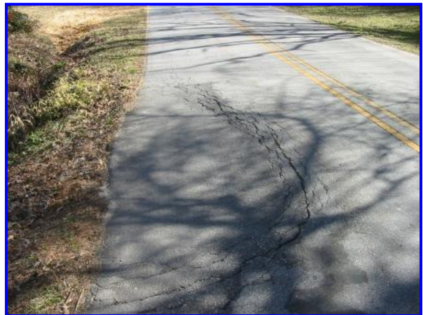
Figure 5.10: Sinking Asphalt on Long John Drive.
